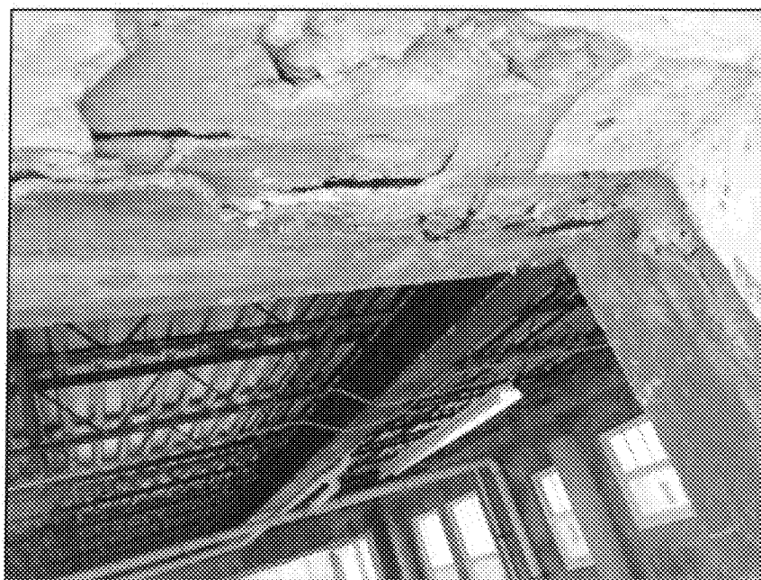
Photograph Number # 6 Description: Corroded and spalling concrete.
