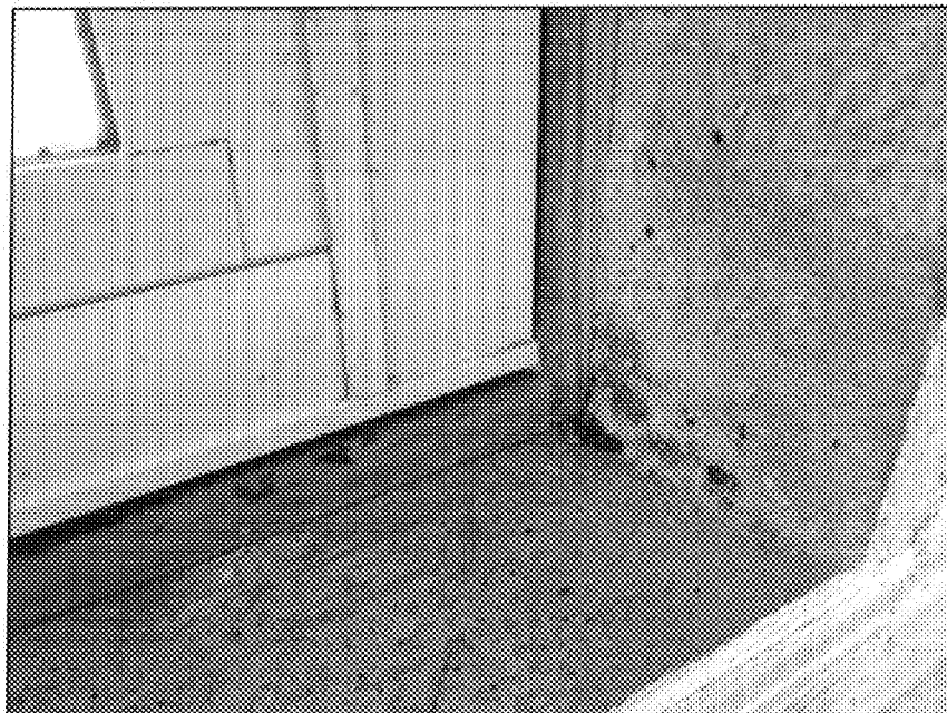
Photograph Number #2-Leak Location Description: Water between wall and buck.
