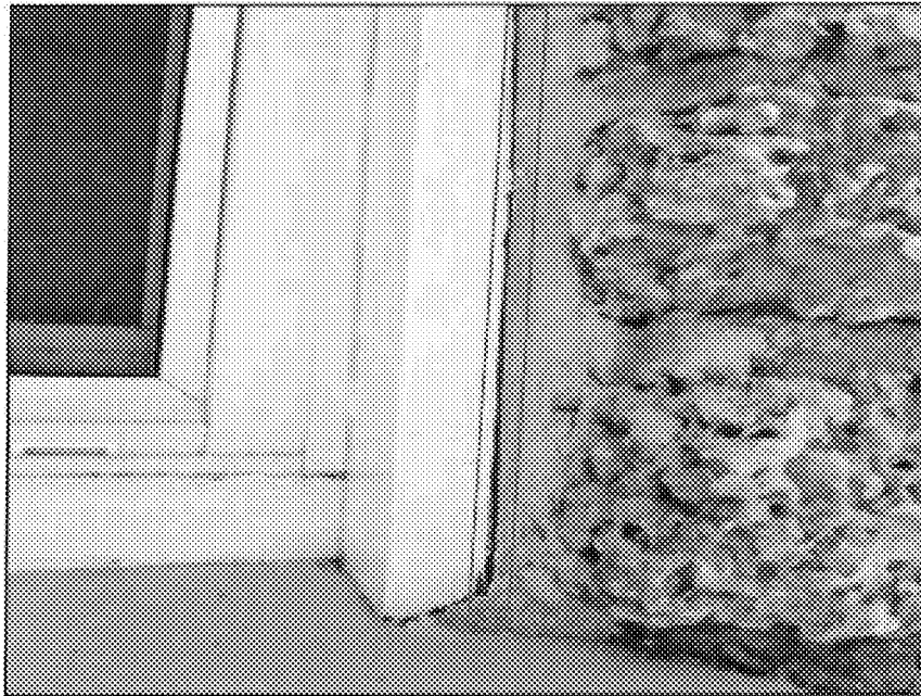
Photograph Number #1-Test Location Description: Cavity between wood buck and coral wall.
