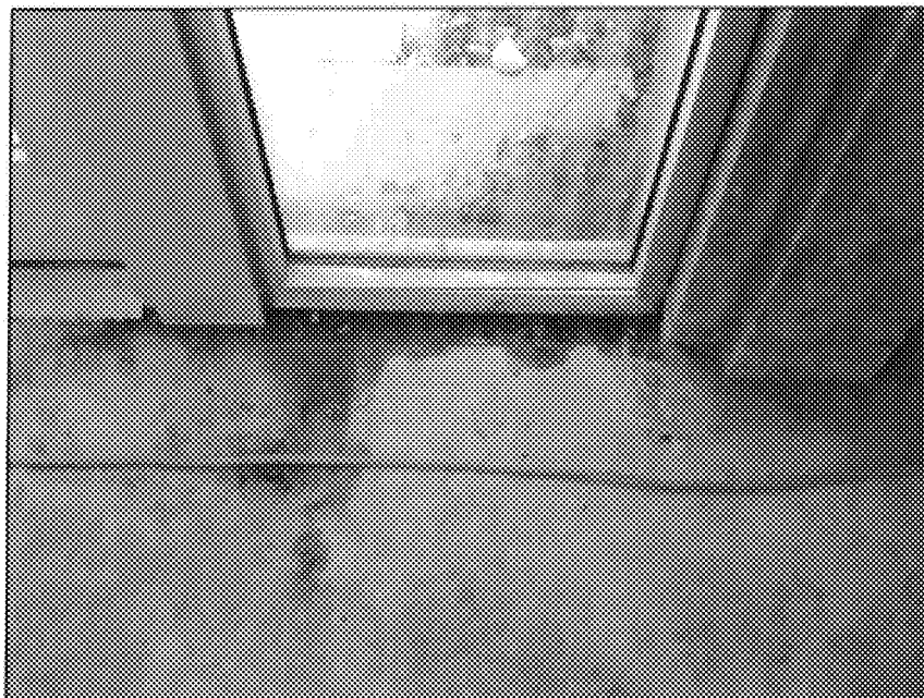
Photograph Number 14 Description: Water migrating between sill and frame.
