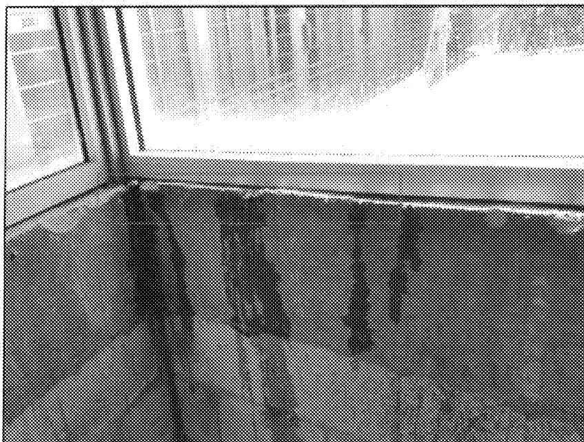
Photograph Number # 10 Description: Water entering sill of window.
