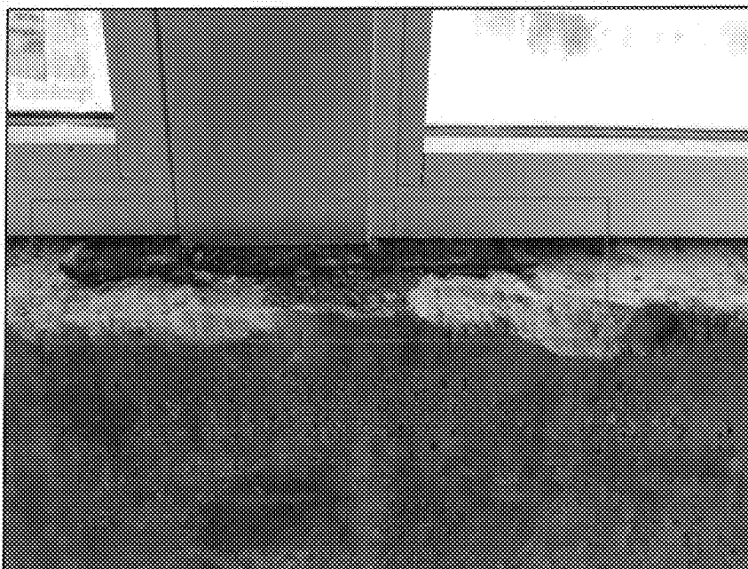
Photograph Number 12 Description: Water entering sill of window.
