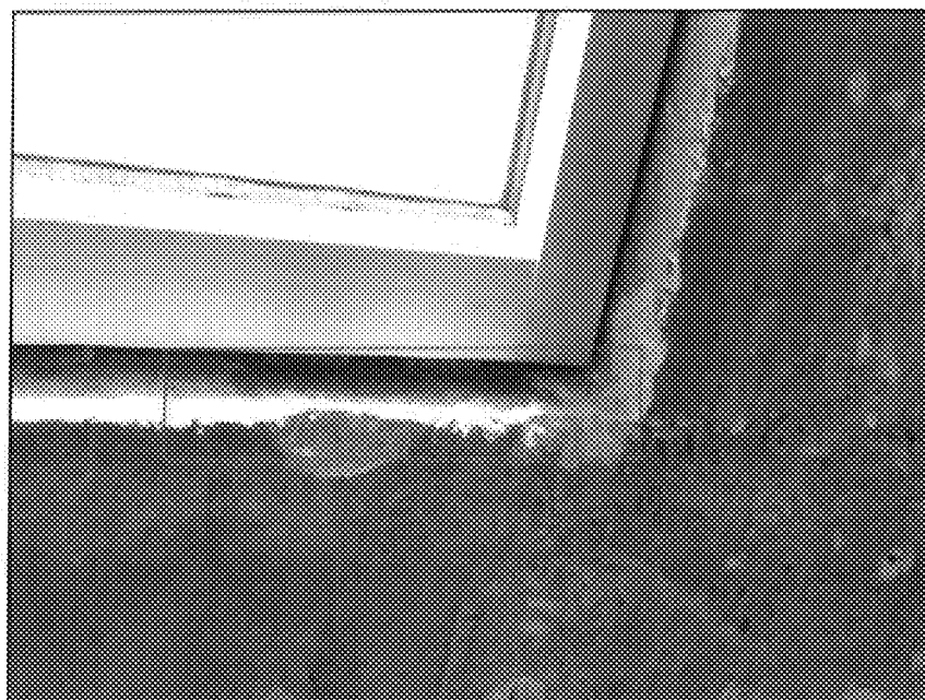
Photograph Number 11 Description: Water entering sill of window.
