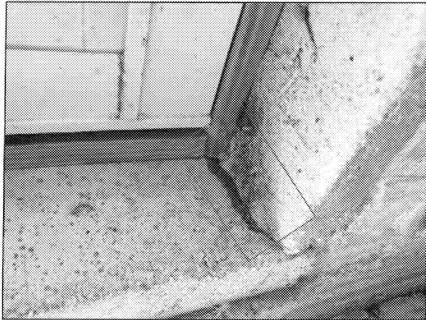
Photograph Number #4-Leak Location Description: Water between buck and wall.
